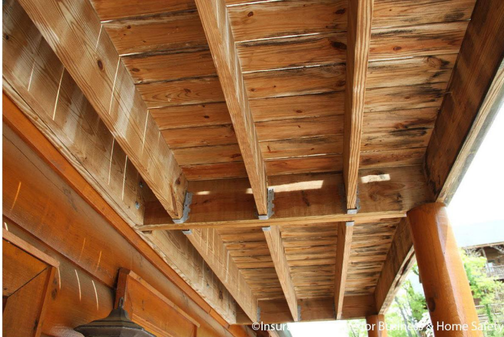
Figure 10. The under-deck structural support system in a deck will trap heat in the same way as under-eave open-frame construction.
