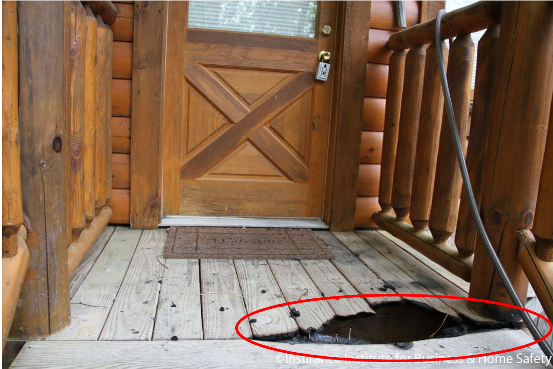
Figure 5. Evidence of likely ember ignition on an entry deck (circled area).
