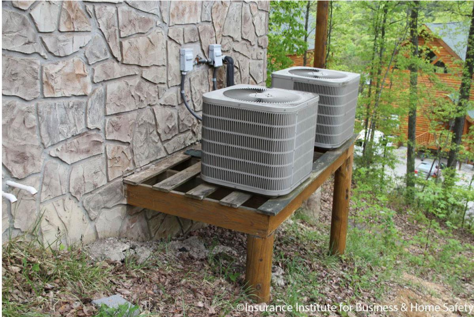
Figure 11. Small platform decks were used to support air conditioning units.
