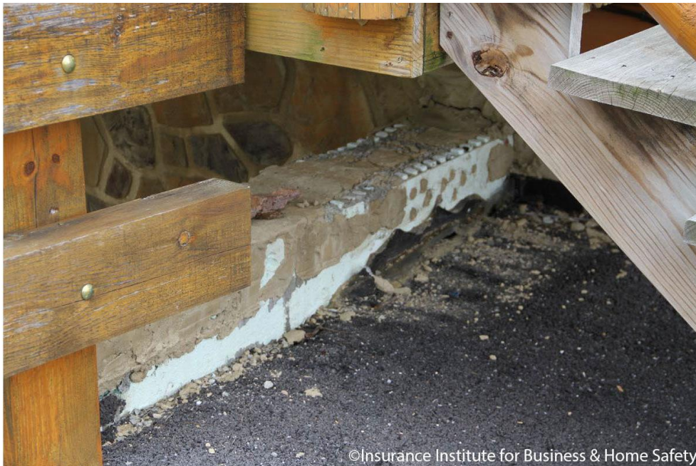
Figure 12. Rigid foam insulation board used on the outside of this concrete form will be vulnerable to direct ember ignition.
