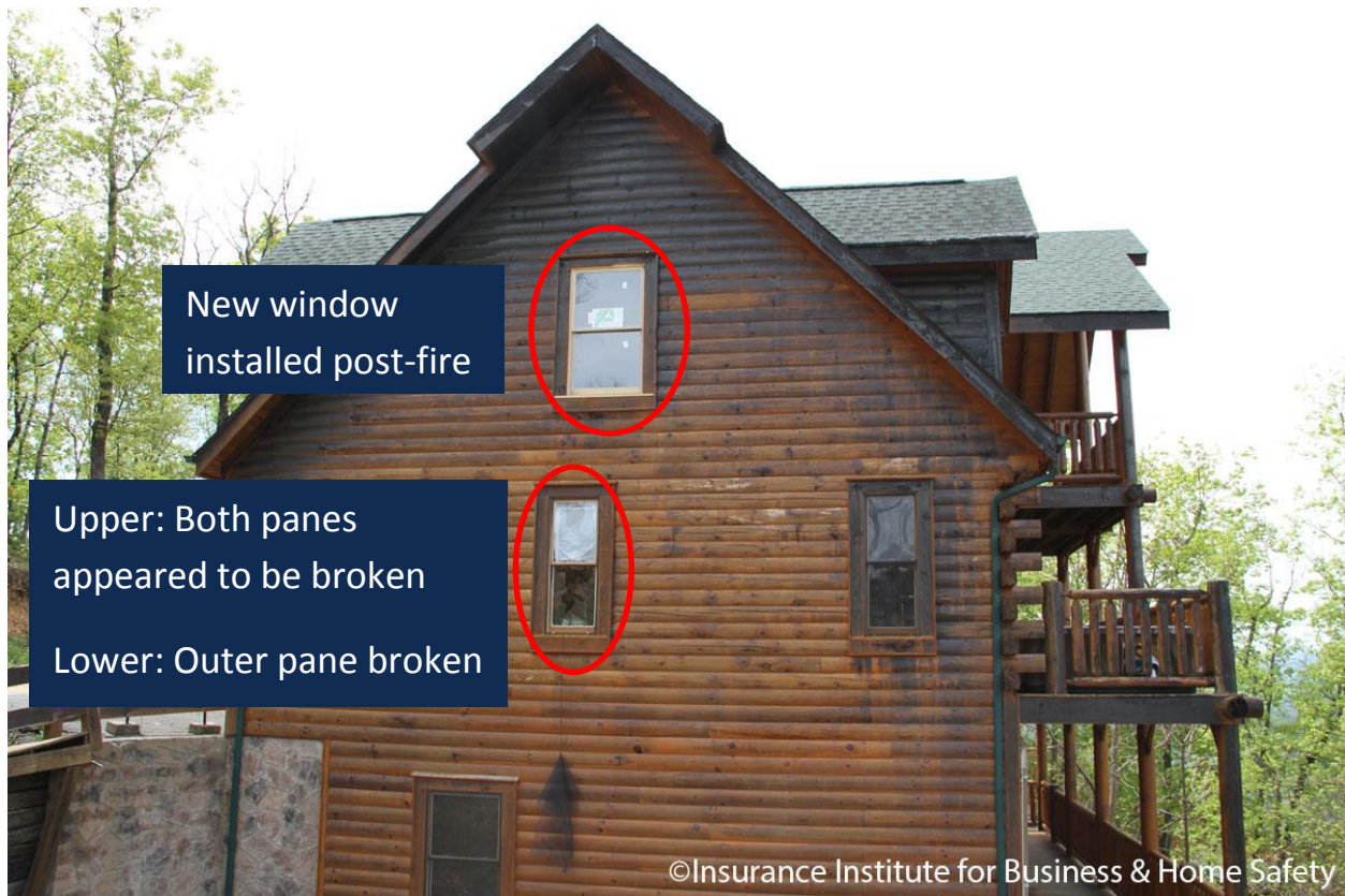
Figure 9. Radiant heat exposure that resulted in glass breakage in windows and scorch to the siding, particularly near the under-eave area on the rake end of the cabin.
