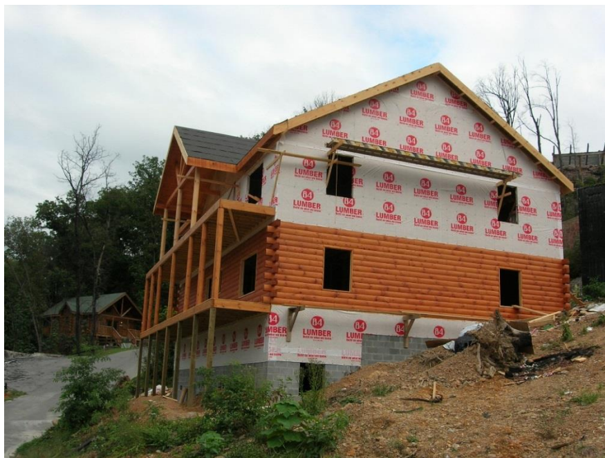
Figure 7. Common construction at Black Bear Ridge Resort consisted of log-wall construction on one level and wood-frame construction on other occupied levels, as shown in this photograph of a cabin being re-built after the Black Bear Cub fire. Note the concrete masonry unit (CMU-block) walls used for the foundation. Photo credit: Leon Konz, Wildfire Mitigation Specialist, Tennessee Division of Forestry
